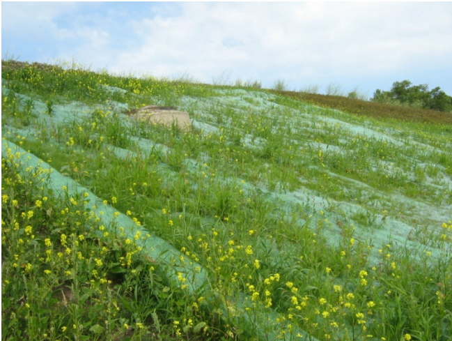
Photo 2 - Looking northeast at edge of repair area by MH7. Light green is reinforcement matting. Good vegetation growth below mat.
