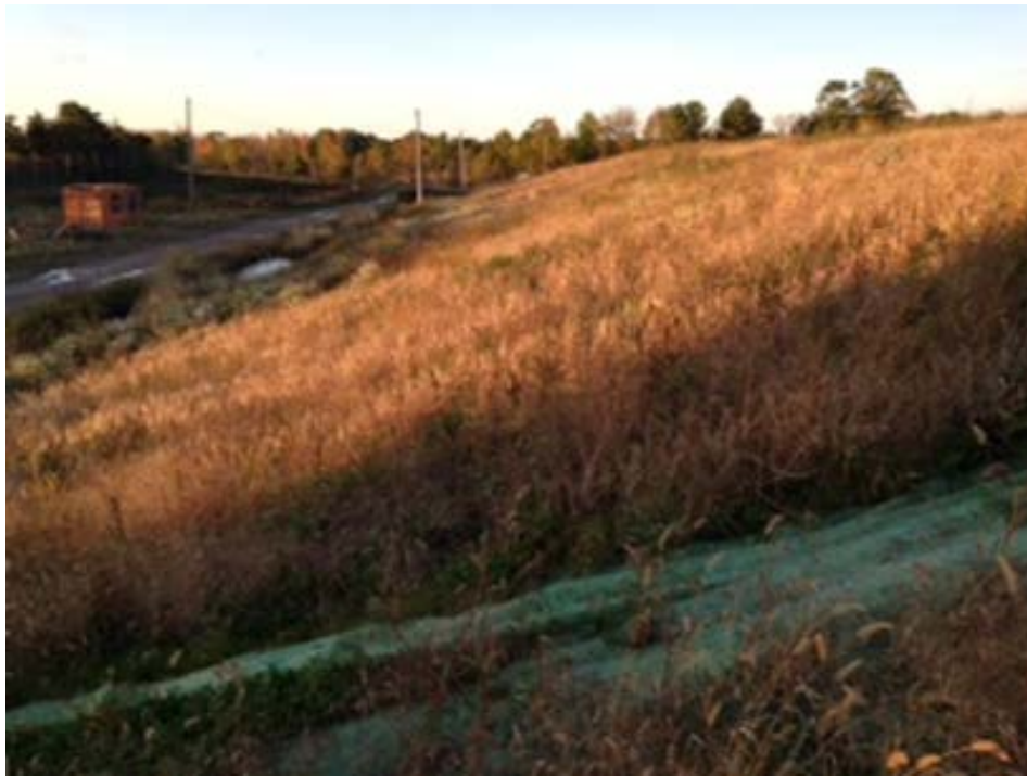
Photo 7 – at manhole on the northeast side looking south. Strong vegetation growth no signs of erosion
