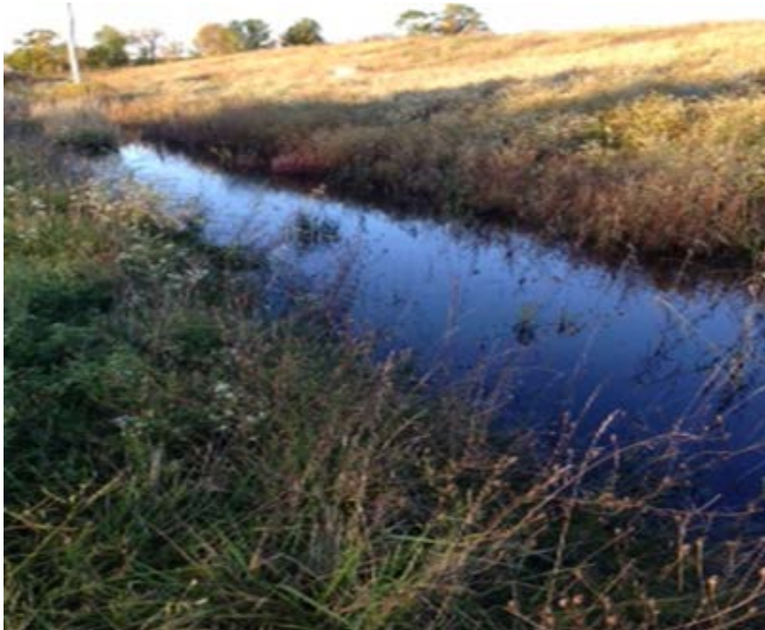
Photo 4 – between south end manhole and middle manhole looking south ditch filled with water culvert blocked (will be cleaning culvert ends out Mid Oct 2014)
