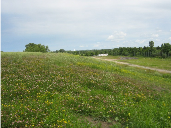
Photo 1 - From southwest corner of EIA looking north. Shows vegetation growth in cover. In foreground is the edge of the repaired area.
