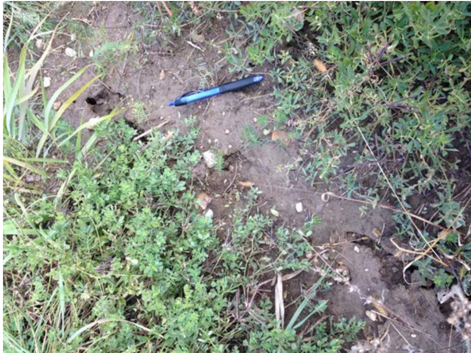
Photo 3 – Minor cracks at area of weak vegetation growth on east sideslope
