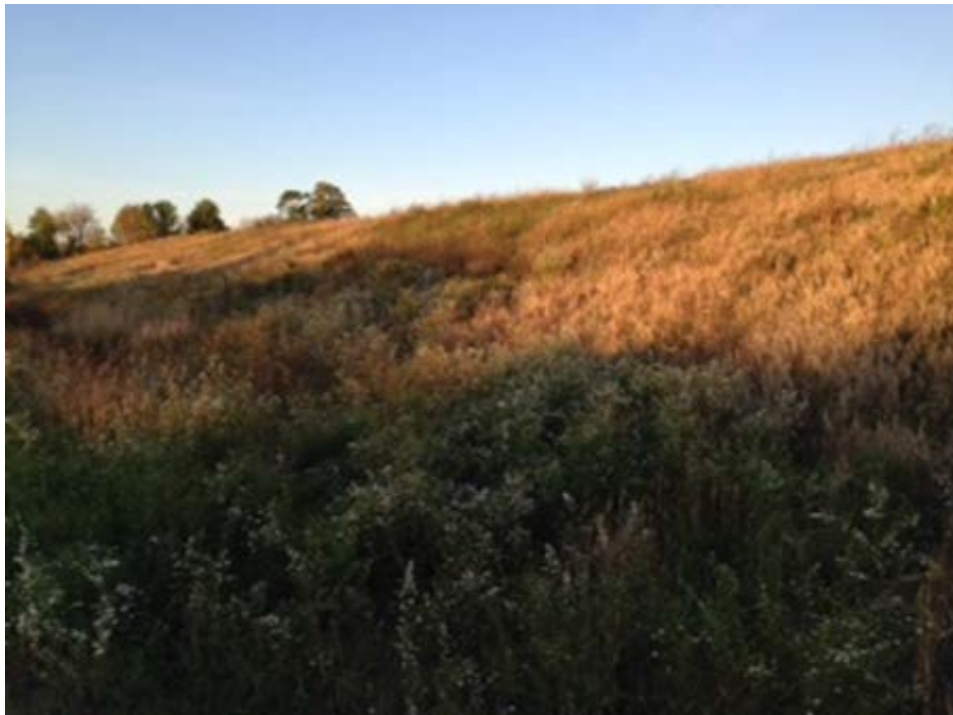
Photo- 9 at the northeast corner looking southwest up the slope. Strong vegetation growth no signs of erosion.
