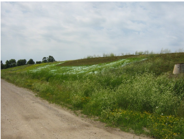
Photo 3 - At northeast corner of EIA looking southwest. Show strong vegetation growth along the slope.
