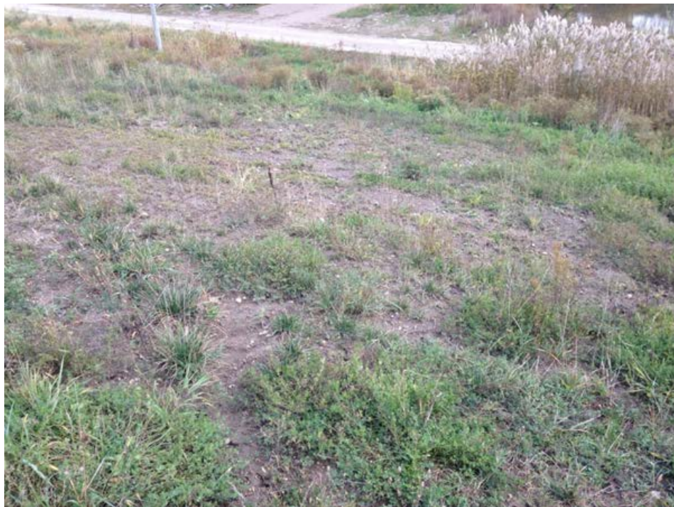
Photo 2 – Poor vegetation growth on east sideslope, near southeast corner
