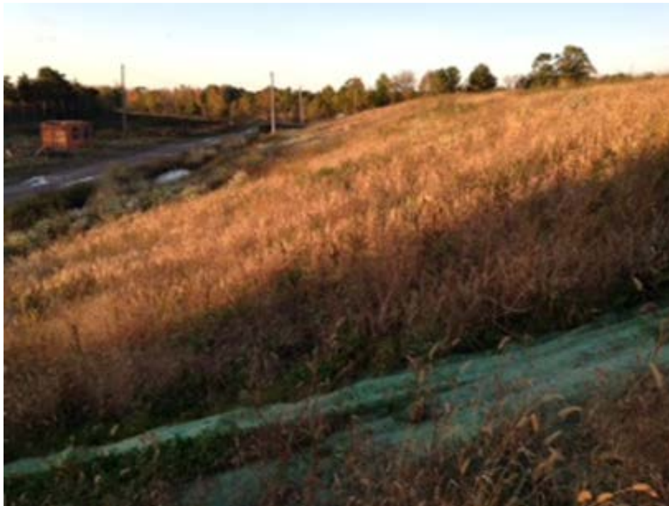
Photo 8 – At manhole on the northeast side looking south. Strong vegetation growth under and through the matting no signs of erosion. Light green is reinforcement matting
